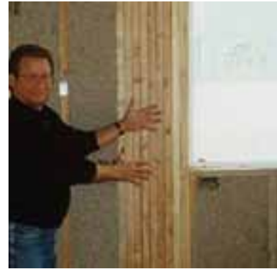
Figure 2 Where one stud is good, two must be better, and 9 must be the ultimate. This is MVE — minimal value engineering.
