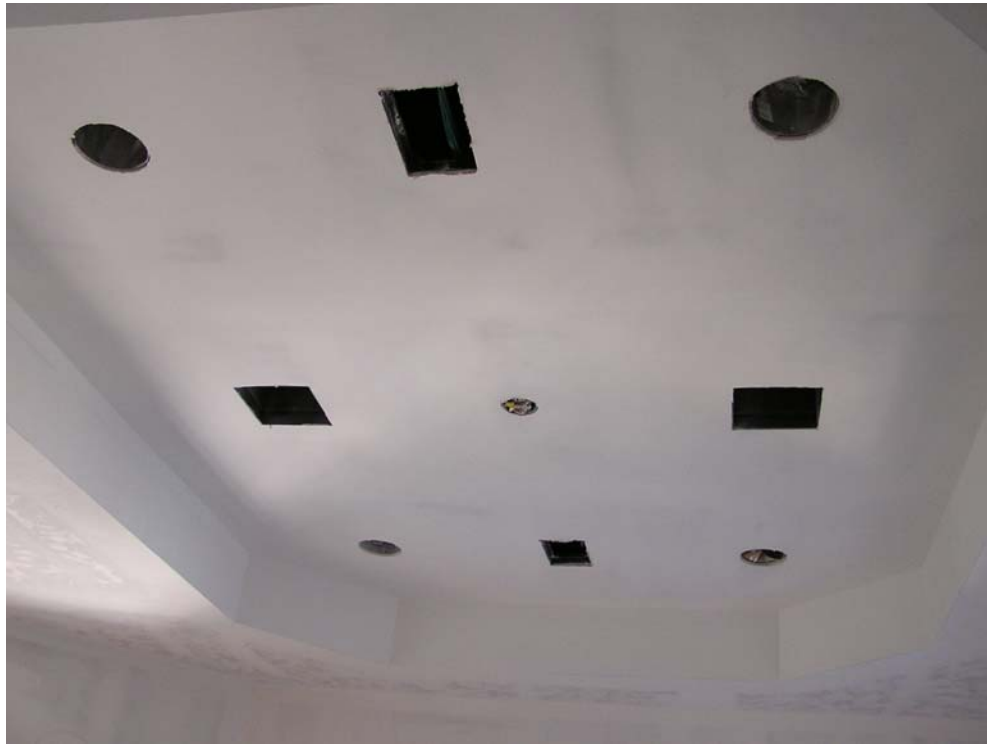
Photograph 1: Ceiling Penetrations – “Swiss Cheese Services”
